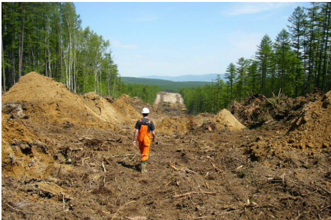
Roads being built for the Sakhalin II are the first incursions into forests. Image: Pacific Environment
